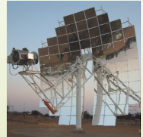
A solar Dish/Stirling generation plant.
